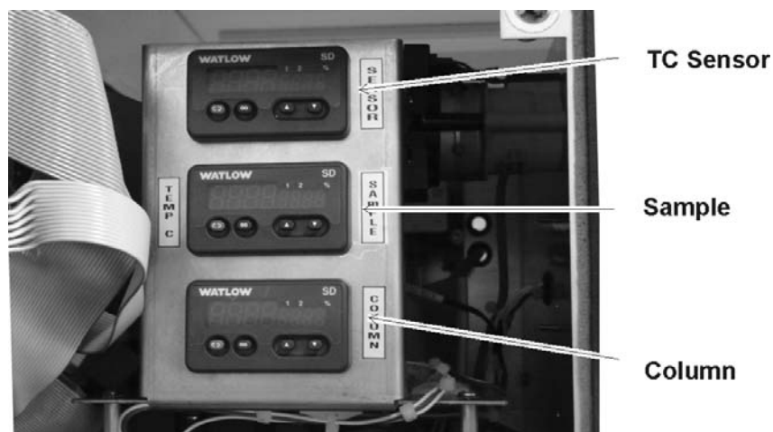
Figure 2-2: Internal Temperature Controllers
